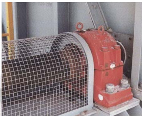
Ventilator drive unit
