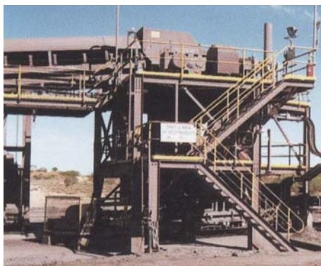
Conveyor plant drive unit
